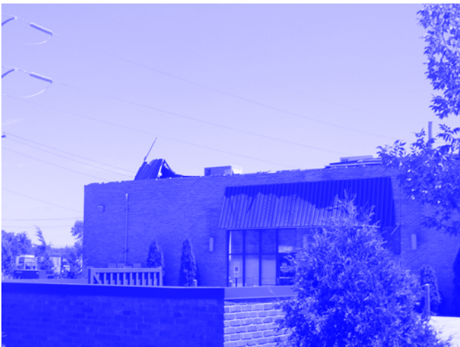
Photo of tornado damage provided by the National Weather Service.
